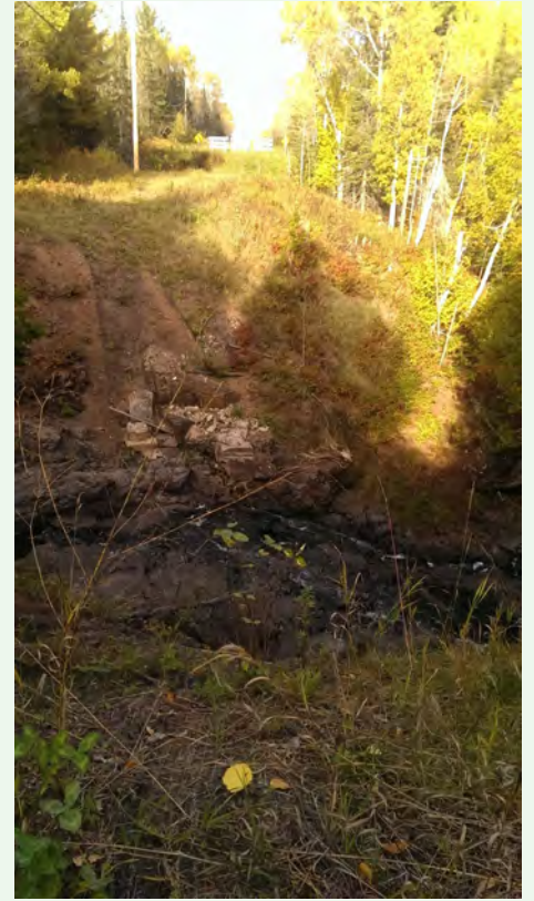
Missing bridge along Old North Shore Road
